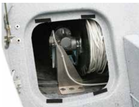
Winch unit installed in Dynamic
